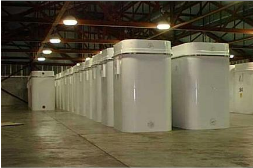
Figure 2-4: DSC Storage Building (Phase I) – Interior
