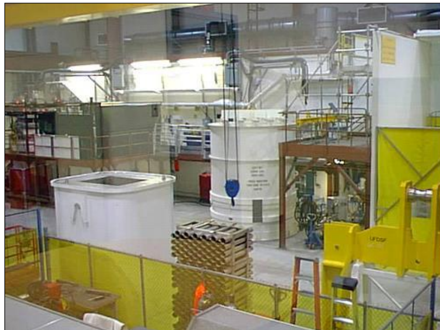
Figure 2-9: DSC Processing Building (Phase I) – Interior
