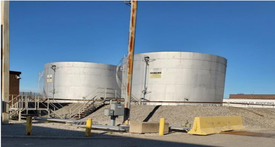
Figure 12 PNGS-A Standby Generator Oil Tanks
