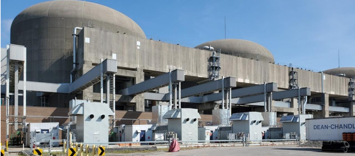
Figure 11 PNGS-A Standby Generators
