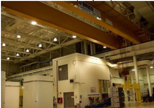
Overhead Crane (Step 12)
