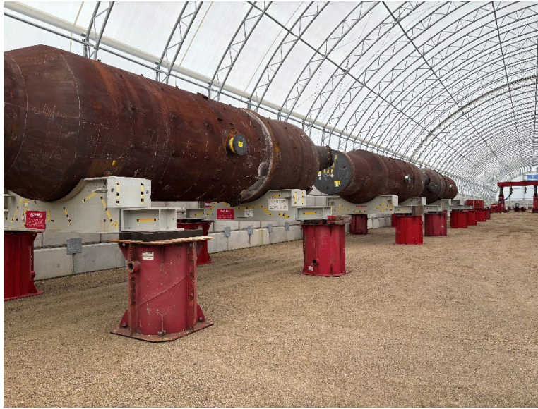
Figure 19: Steam Generators inside MPSB
