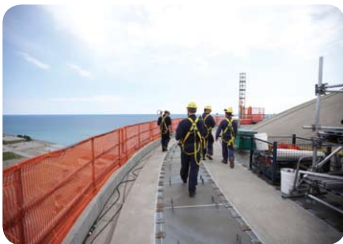
Darlington Outage staff on top of the Vacuum Building: to prepare for the outage, hoisting and rigging equipment were brought in, and a temporary elevator was erected to allow crews to access the roof.
