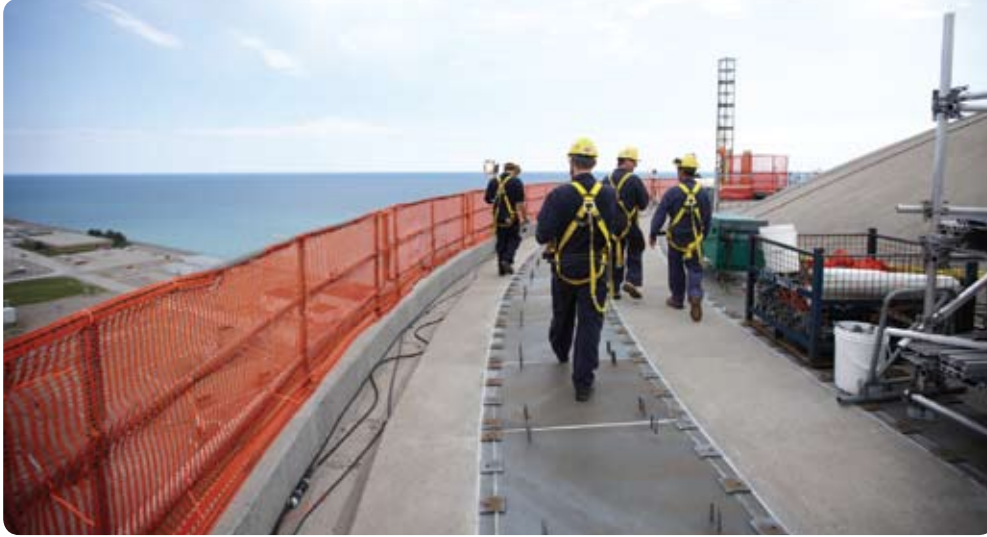
Outage staff on top of the Vacuum Building: To prepare for the outage, hoisting and rigging equipment were brought in, and a temporary elevator was erected to allow crews to access the roof.
